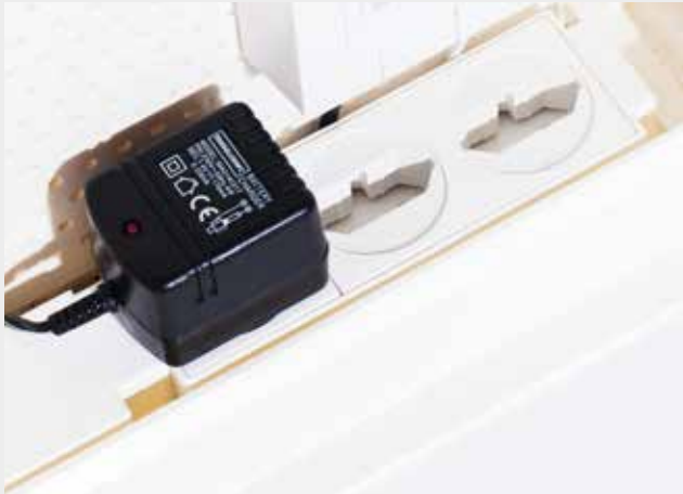
The hardware components are fixed to the plastic equipment racks, potential-free, and supplied from the mains via the triple socket.
